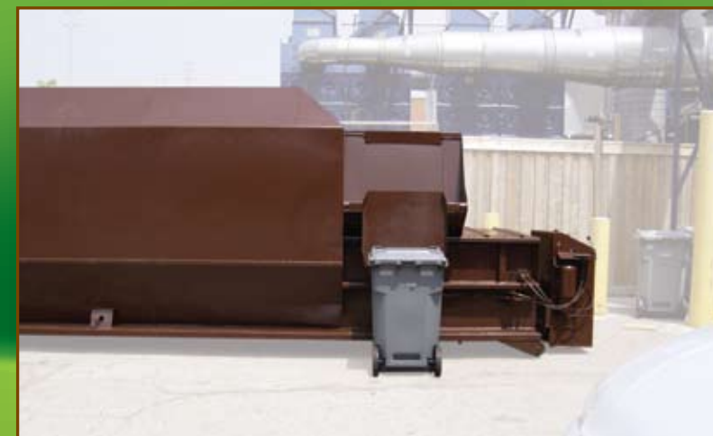
Enclosed Hopper with Cart Dumper
